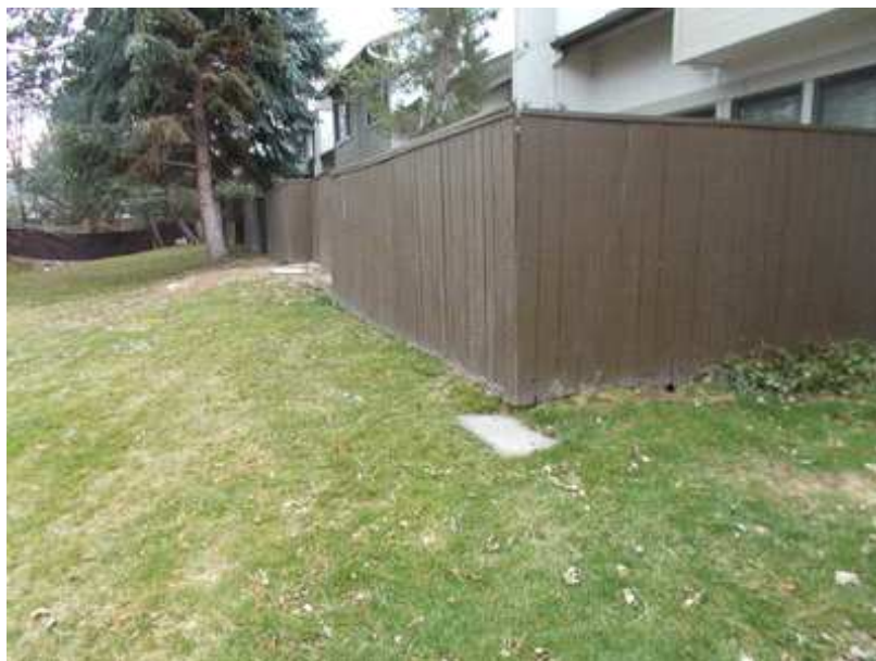
The Board of Directors may want to consider moving the grass away from the Patio Fencing so that water from the sprinklers does not damage the fencing.
