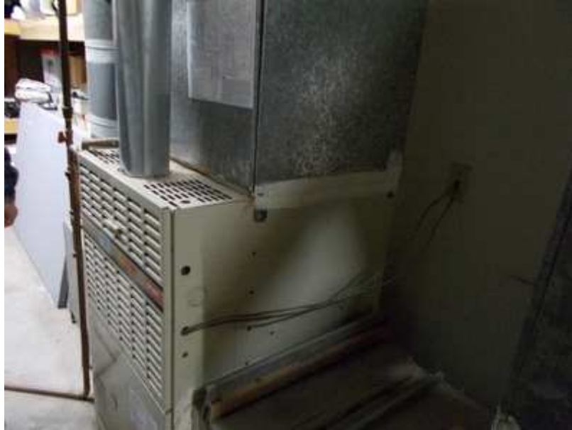
There are 2 HVAC Units for the Clubhouse. Maintenance and Replacement have been included in the Study.
