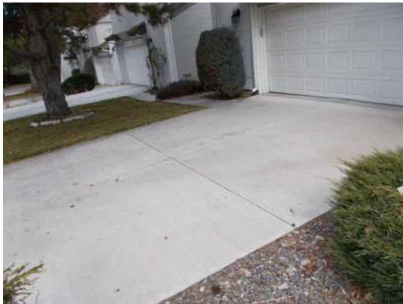
The Driveways are maintained by the Homeowners Association. Replacement is included in the Common Area Concrete Allowance.
