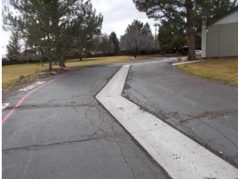
Removal and Reconstruction of all Asphalt Roads and Concrete Drainage Swales have been done in phases.
