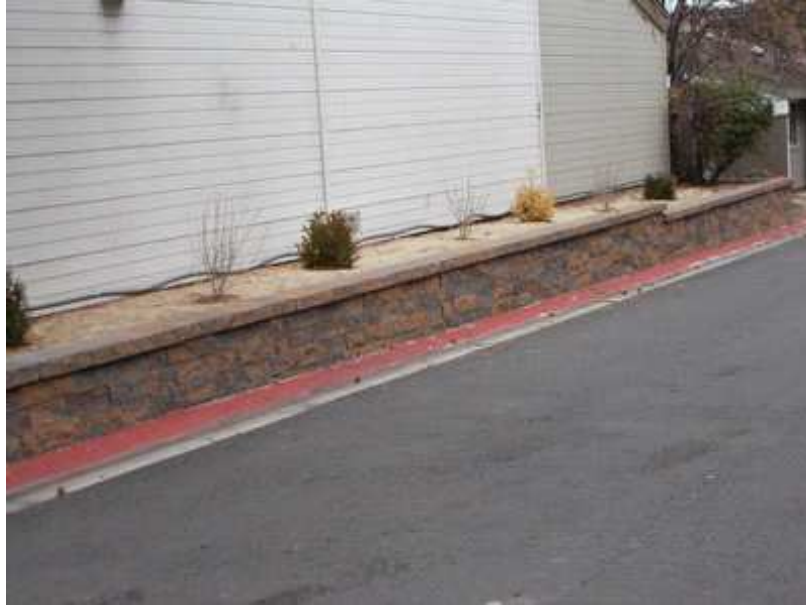
Retaining Walls were replaced in 2018, future replacement has been included in the Study.
