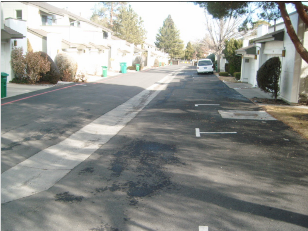
The Asphalt Removal and Replacement and Concrete Drainage Swale Replacement has been scheduled in Phases to be done within the next 4 years.
