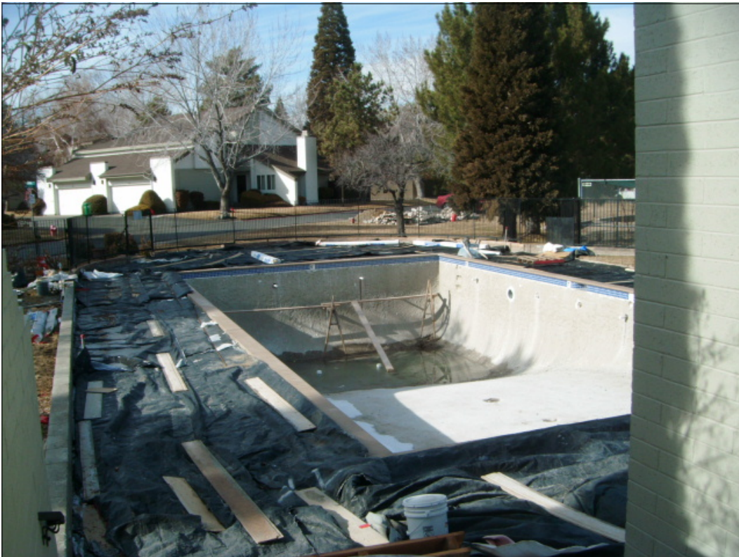
The Pool is being completely rebuilt. All Pool Components and new estimated useful lives have been included in this Study.
